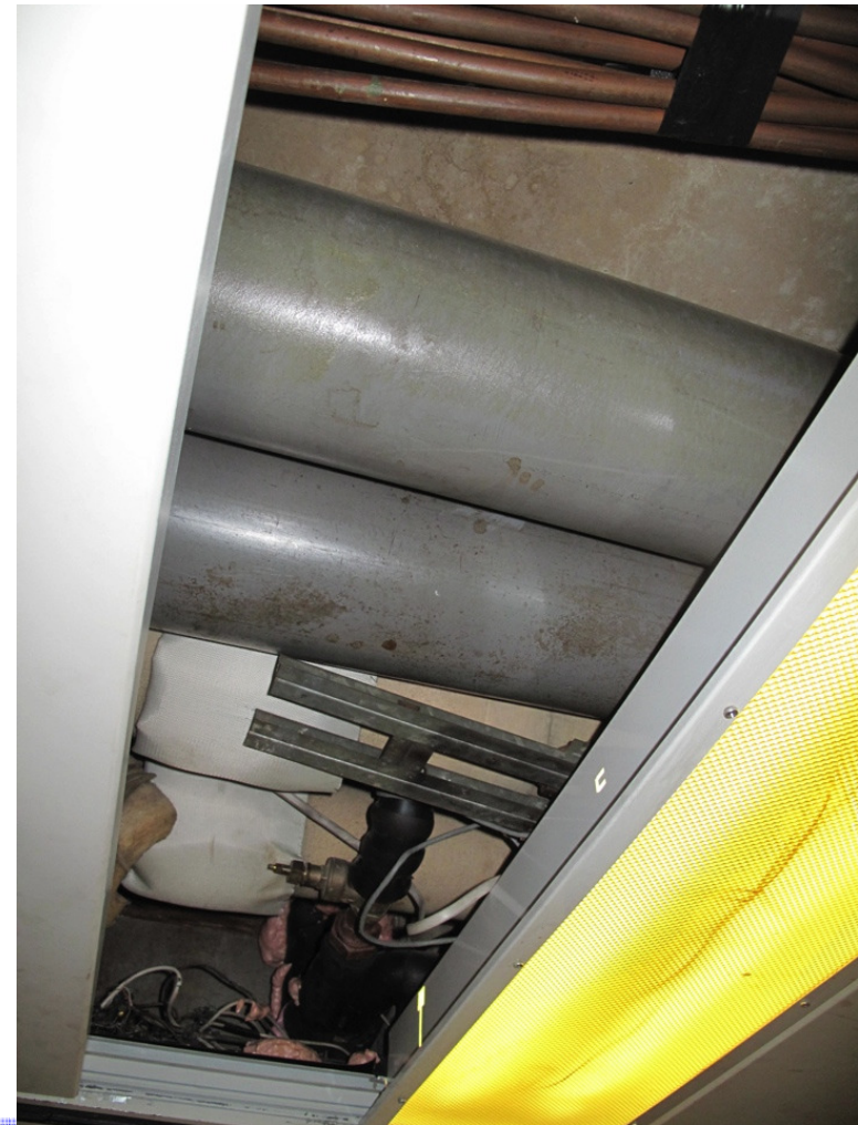
Services within the common access corridor ceilings
