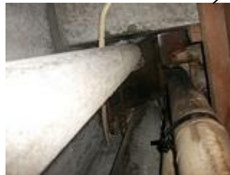
Cement boarding at pipe penetration point
